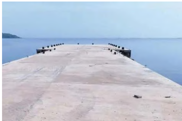
A photo of the ferry ramp at the Sh500 million Homa Bay pier that is being rehabilitated to serve as vital maritime link to Kisumu, Kendu Bay, Mbita, Uganda and Tanzania hubs.
