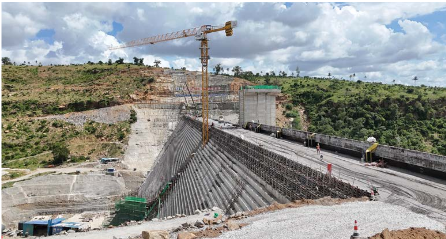
Aerial view of the Mwache Main Dam, currently at an advanced stage of construction, marking a major milestone in the implementation of a long-term solution to address water shortages in Mombasa and the Coast region. PHOTO: CHARI SUCHE
