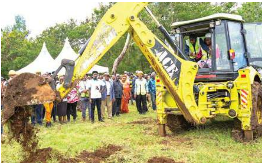
Embu Governor Cecily Mbarire operating a backhoe loader to mark the groundbreaking of Rupingazi-Weru Irrigation Scheme in Mbeti South Ward, Mbeere South Constituency. The Sh69.9 irrigation project targets to benefit over 360 households covering 150 hectares.
