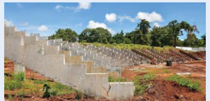
The current state of the Kamariny Stadium, which is under construction to host Mashujaa Day. PHOTO BY JUNE JEBET
