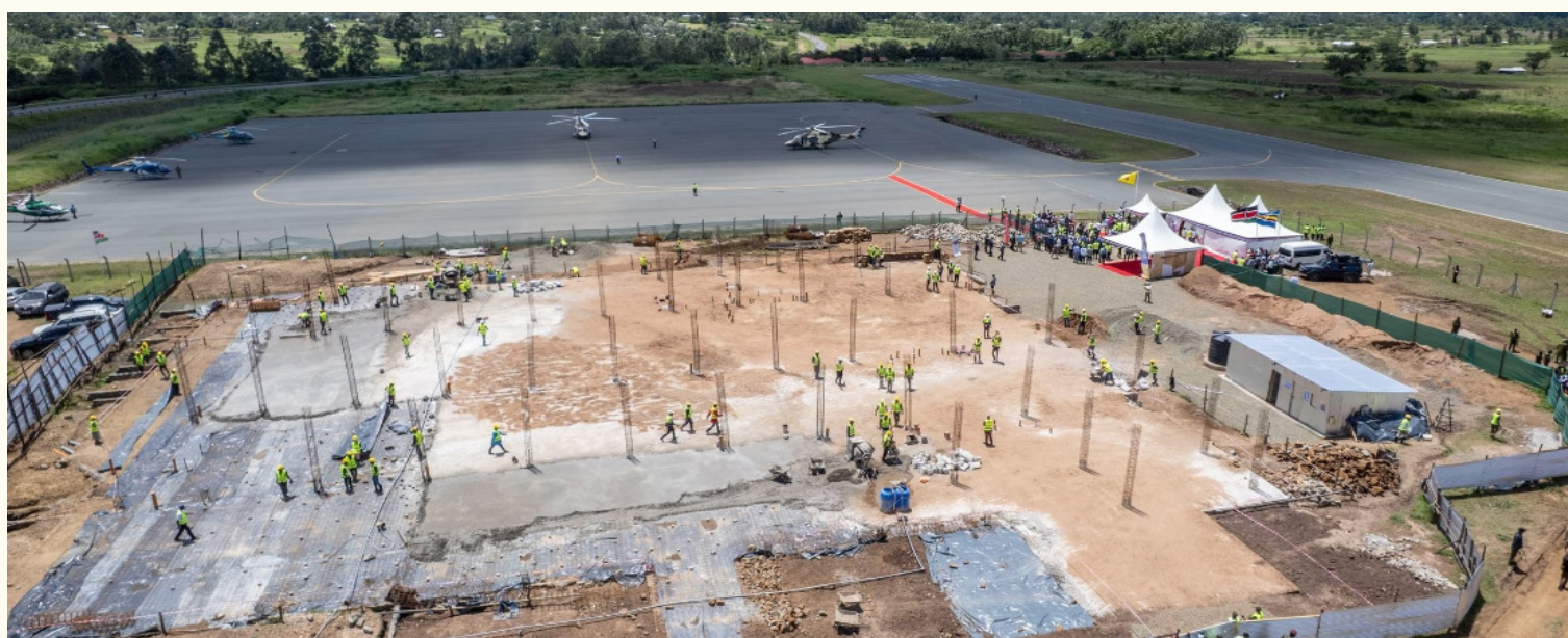
An aerial view of Lichota Airstrip in Suna West Constituency, Migori County. The airstrip is undergoing expansion and modernisation at a cost of Sh280 million, a strategic investment aimed at enhancing regional connectivity, including links with neighboring Tanzania and boosting tourism to the Maasai Mara National Reserve.
