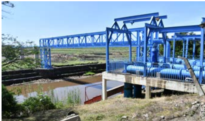
A section of the Ahero Irrigation Scheme Pump station.
