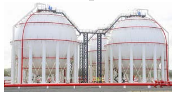
Construction of the ultra-modern LPG firm Lake Gas in Vipingo in its final stages.
