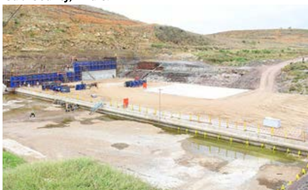
Construction of the Mwache lower check dam in progress in Kinango Sub-County, Kwale.
