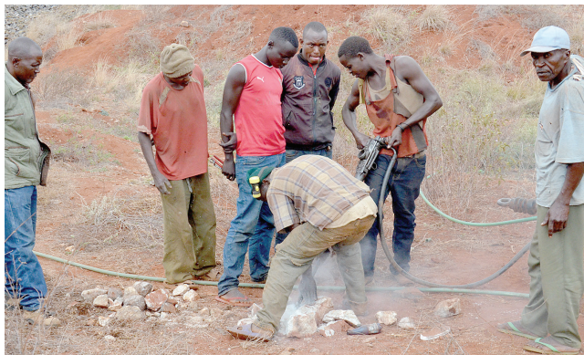
A section of artisanal miners at Chawia in Mwatate use a jackhammer, to rip through a rock in search of precious stones.
