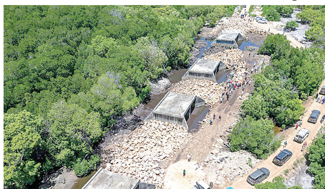
An aerial view of the iconic Funzi causeway project in Kwale taking shape at an unparalleled speed to boost connectivity and safety.
