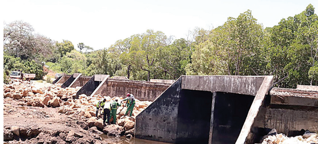
Construction works of the new Funzi island causeway project in Kwale gathers pace.
