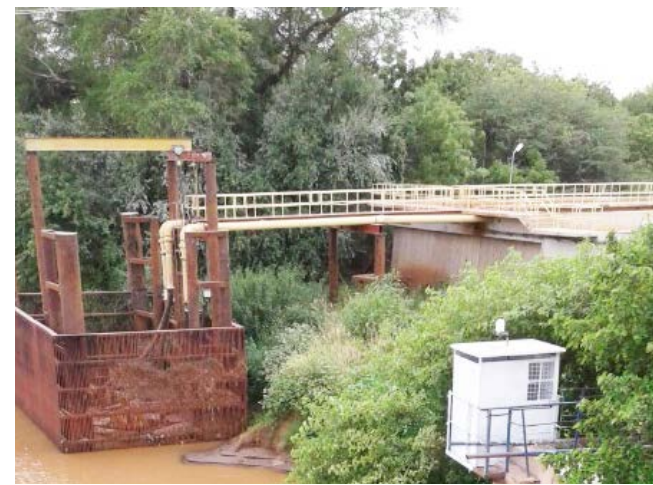
Telemetric station equipment housing that monitors water abstraction: Photo: WRA.
