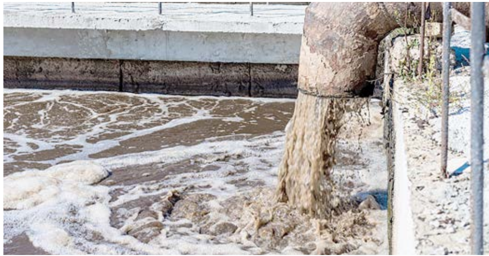
A waste water recycling plant. Nakuru County Government is seeking Israel waste recycling companies to invest in circular economy solutions for zero waste
