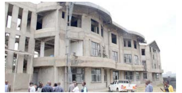
A section of the incomplete Lake Victoria Basin Commission (LVBC) headquarters building in Kisumu.
