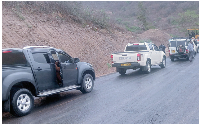
A section of the 54-km Mto Mwa-godi-Dawida-Mbale-Wundanyi-Bura road in Taita-Taveta County that is nearing completion.
