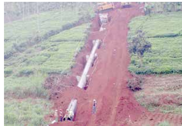
Installation of new water line from Ndakaini to Kirogo water treatment area going on.
