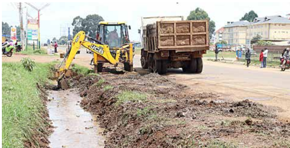
Ongoing opening of drainages in readiness for conferment of Eldoret to city status
