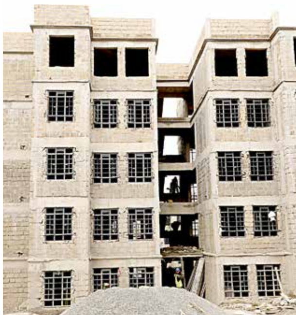
Affordable housing units under construction in Elburgon, within Molo Sub-County. Governor Susan Kihika has announced that the affordable housing projects in Molo and Bahati Sub-Counties are 60 pc complete. Photo by Anne Mwale
